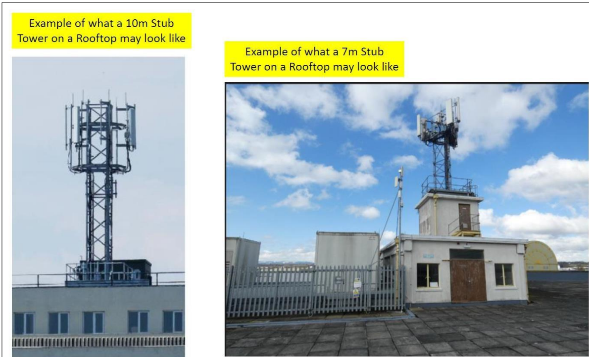
Image 2 - Examples of a 10m & 7m High Stub Tower on a rooftop ( Not to scale and only for reference ).
